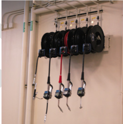
Figure 4-51 Fluids Distribution System
