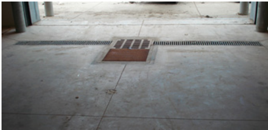
Figure 3-3 Trench Drain in VMS Workbay, Fargo, North Dakota
