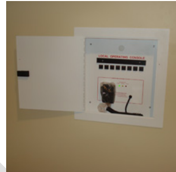
Figure 2-7 Local Operating Console (LOC) for Mass Notification
