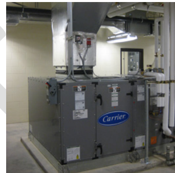
Figure 3-11 Air Handling Unit
